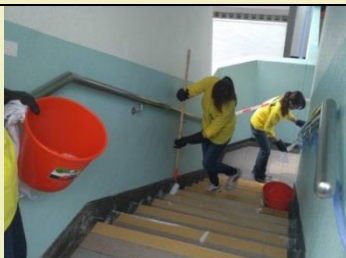
(5) Use appropriate tools to apply F222p. Continuously check and resupply F222p to ensure that the surface will not dry out.
