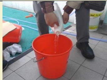
(4) Pour out appropriate amount of LABond STEPGUARD F222p (Do not dilute, please refer to the coverage for each kind of surface)
